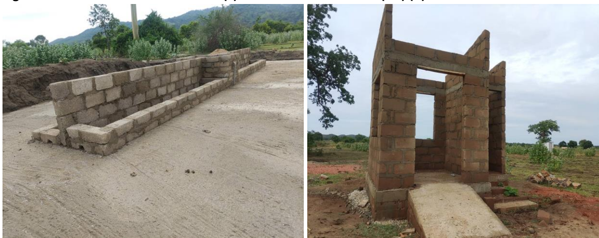
Figure 4: Photos of Cattle trough (L) and Guard house and toilet (R) under construction
