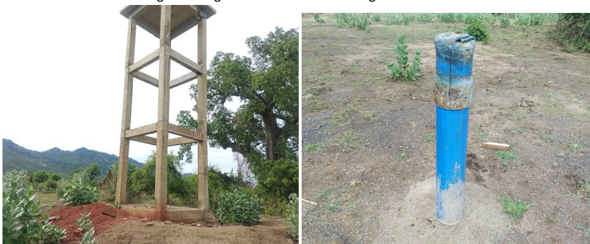
Figure 3: Photos of Water tank tower (L) and the Domestic Point (PD) (R) under construction
